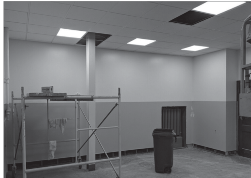
New LED Lighting!
